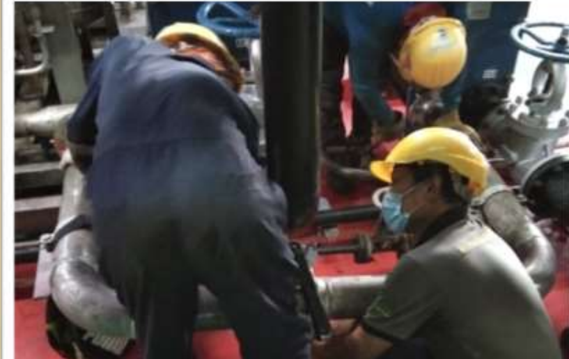
Assy PIPING STATOR COOLING On Site
