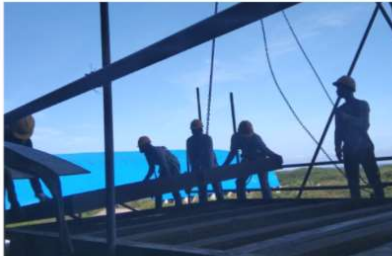
Change FILTER SILLINCER FDF On site
